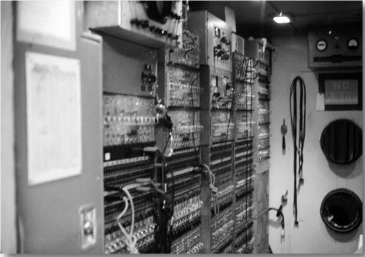
Equipment in one of the Tropospheric Scatter Microwave Communication vans
